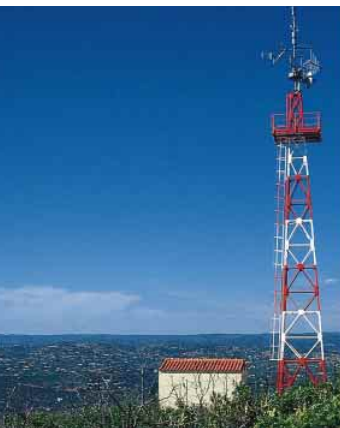
FIG 2 An antenna system of Transmitter Monitoring System SMSA Photo: Pfitzner
